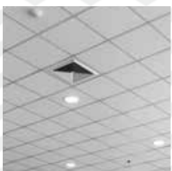
CEILING GRID FALSE CEILING
